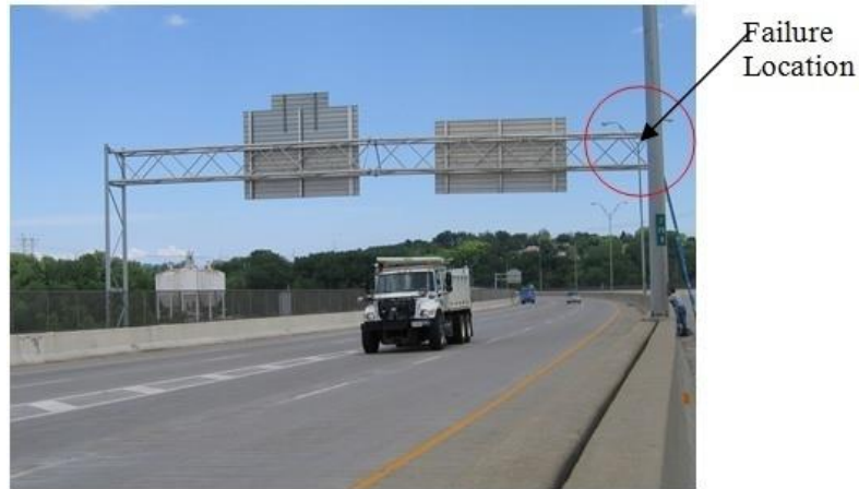
Figure 3. Failure location of the sign support structure.
